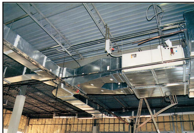
Air handlers (drawing and photo) are tied together in parallel to create four stages of heating and four stages of cooling. This unit serves one of the six zones in the 33,005 ft 2 office.
