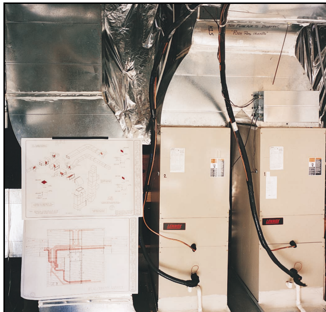
Energy recovery ventilation system heats and cools the house for less than $75 per month.
